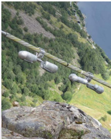
◀ Vibration dampers installed on protection rods.
