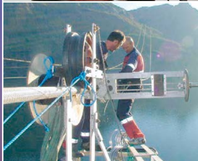
◀ Fjord crossing in Norway Sunnalsfjord: 3 spans, max. 3,670 m span length (436 kN RTS).
