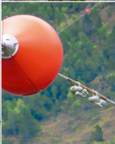
◀ Aircraft warning sphere with installed vibration dampers.
